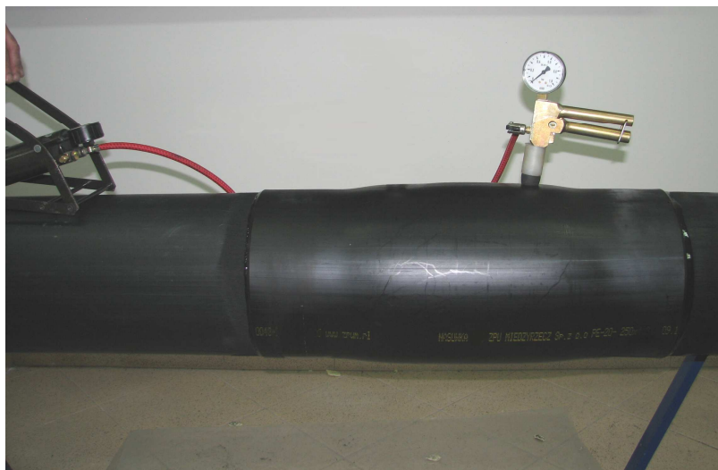
Photo No. 33 Control pressure gauge mounting
